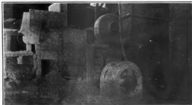
Motor Driven Hammer Mill for Making Ground Lime With Elevator at Right
